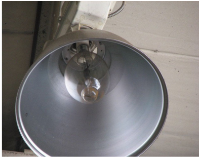
Figure 1: Metal Halide Bulb in Open Fixture
