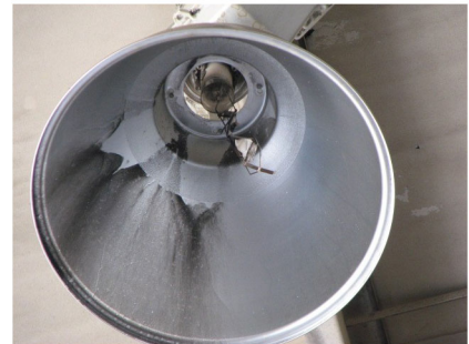
Figure 2: Ruptured Metal Halide Bulb in Open Fixture
