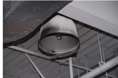
Figure 6: Acrylic Enclosure Failed to Contain Rupture
