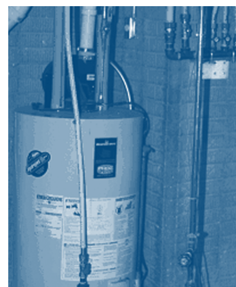
Each of these PCV covered lines is a home run, such as the one shown to the hot water heater.
