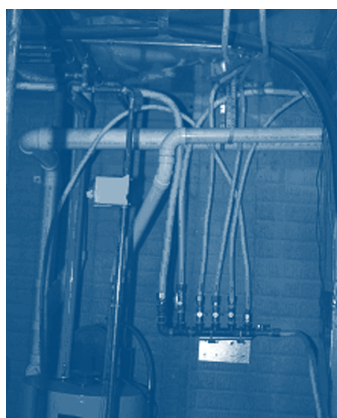
This photograph shows a central manifold for a CSST system. Notice how many gas lines come off the manifold.
